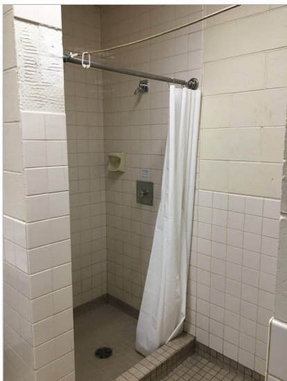
Photo 3.3-2 Men’s Shower in Willow
